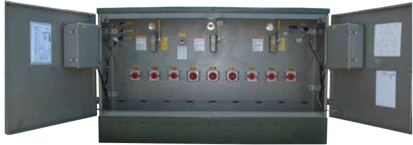
Figure 3. VFI switchgear 6-way unit.
